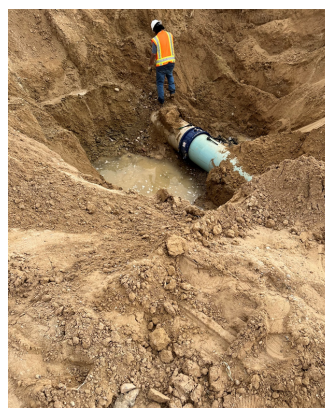
Figure 5. Excavation of large main-line for irrigation into the ASC Farmington during infrastructure repairs.
